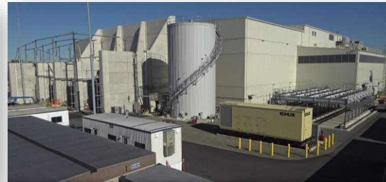
Astoria Converter Station
