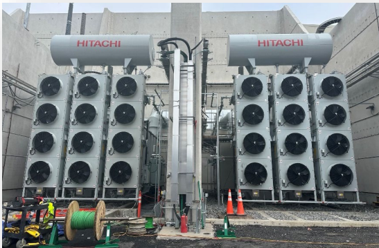
Converter Station Transformer Bays
