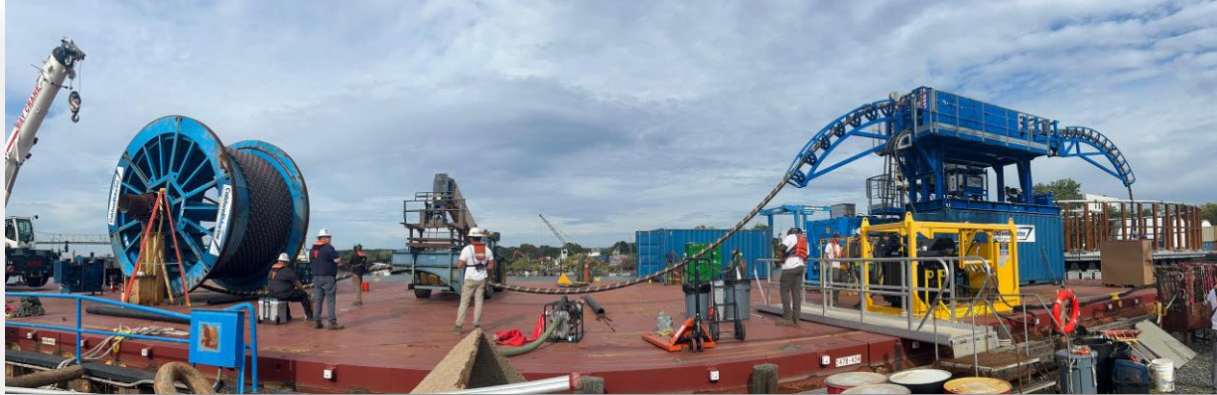
Cable Transpooling, Harlem River
