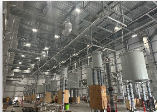
Converter Station Halls Equipment
