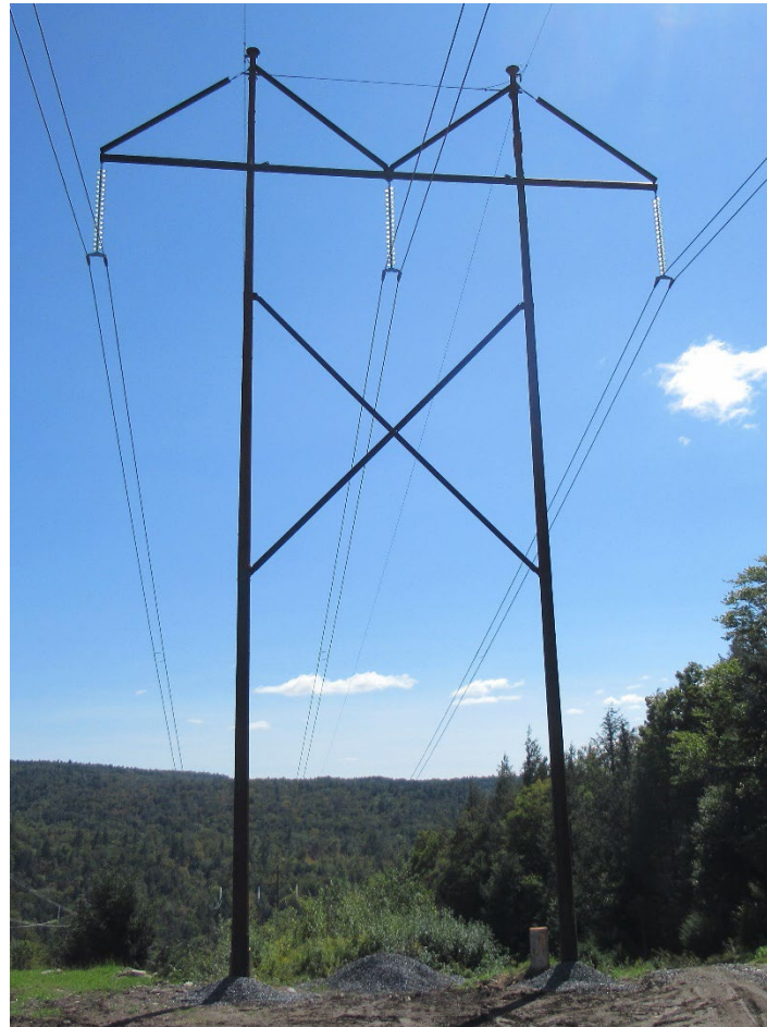
345 kV Steel H-frame
