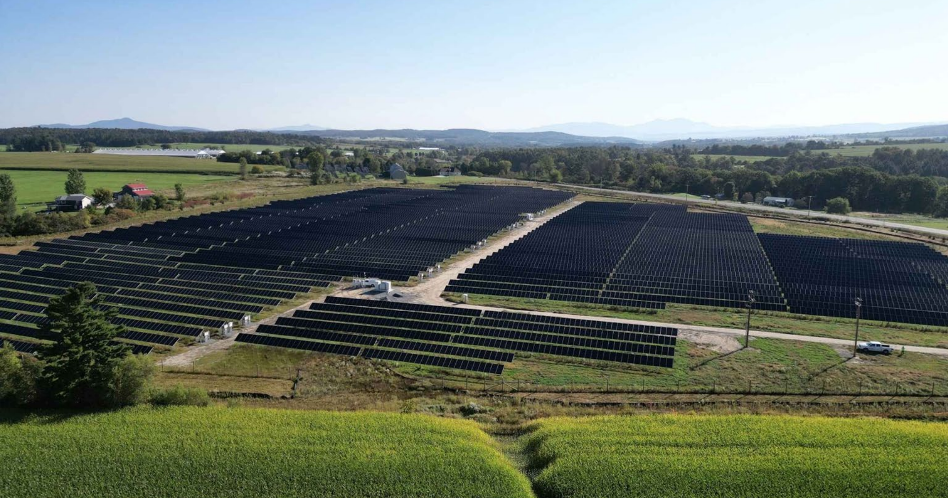
Encore Danyow Road PV Project in Sheldon, VT
